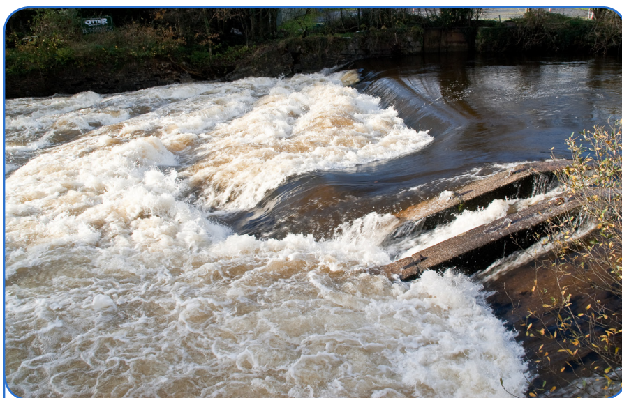
An old form of fish ladder on the River Dart in Devon. As the name suggests, it was built to facilitate salmon going up river to spawn. Measures such as this can help mitigate the impact of small hydro schemes on river habitats.
